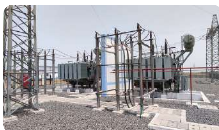
Transformer in a solar site in India
