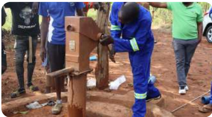
Operator checking a water borehole and its pump
