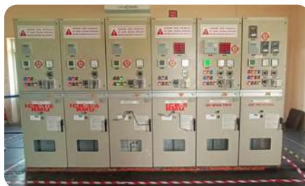
Technical installations of the project
